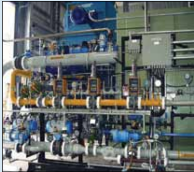
Rack-mounted fuel trains were prepped and wired at the factory
