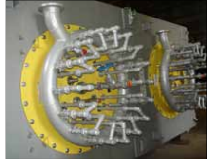
"Each boiler also includes a dual burner, state-of-the-art, low NOx combustion system with rack-mounted fuel trains."
