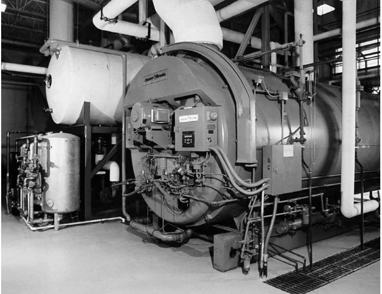
Figure 1-14: Operational Boiler Room
